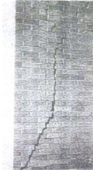
Figure E-2: Structural cracks in masonry
