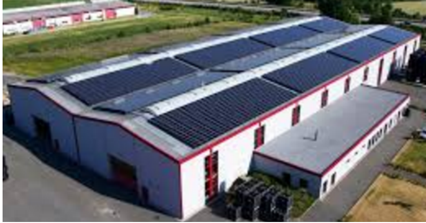
Figure E-22: Roof-mounted solar PV penetration
