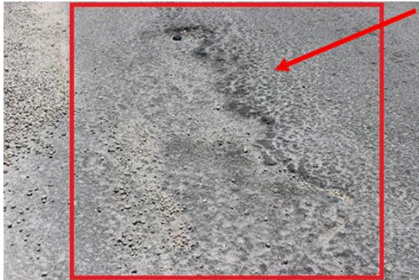
Figure E-5: Degradation modes of roads—surface degradation due to ponding
