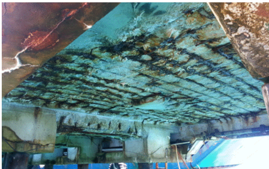
Figure E-12: Example of structural corrosion at wharf
