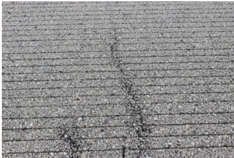
Figure E-8: Runway surface degradation due to cracks
