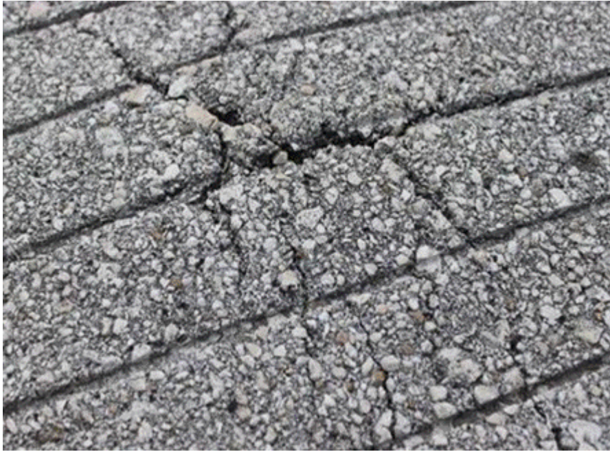
Figure E-10: Runway surface degradation due to volcano cracks
