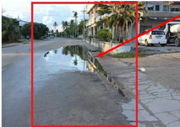
Figure E-7: Degradation modes—clogged drainage sump
