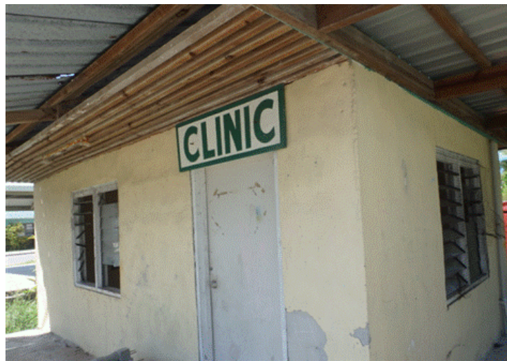
Figure B-14: Recently constructed clinic building in Meneng—roof and windows are at the end of life
