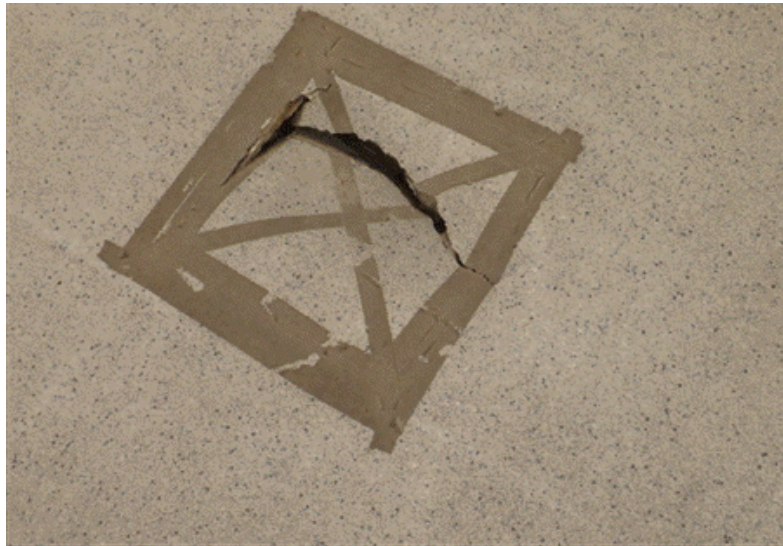
Figure B-12: Poor quality of construction at the new hospital building where low ceilings and flimsy ceiling material is resulting in damage to ceilings
