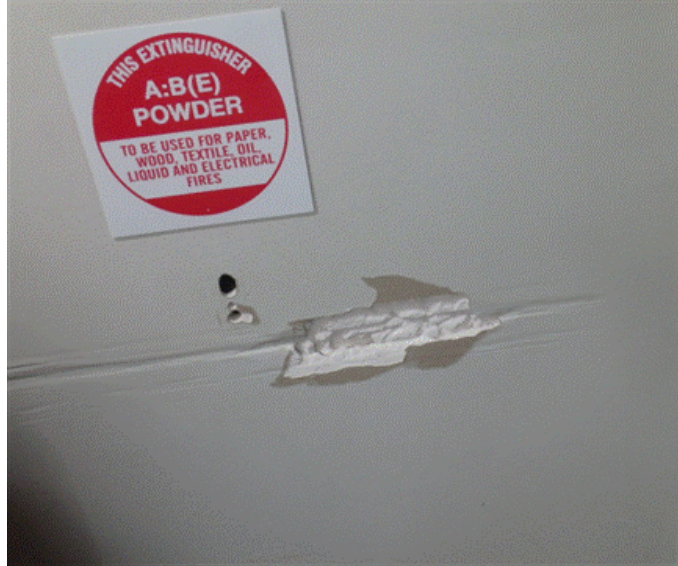
Figure B-9: Poor quality of construction at the new hospital building, showing where the fire extinguisher fell off its mounting
