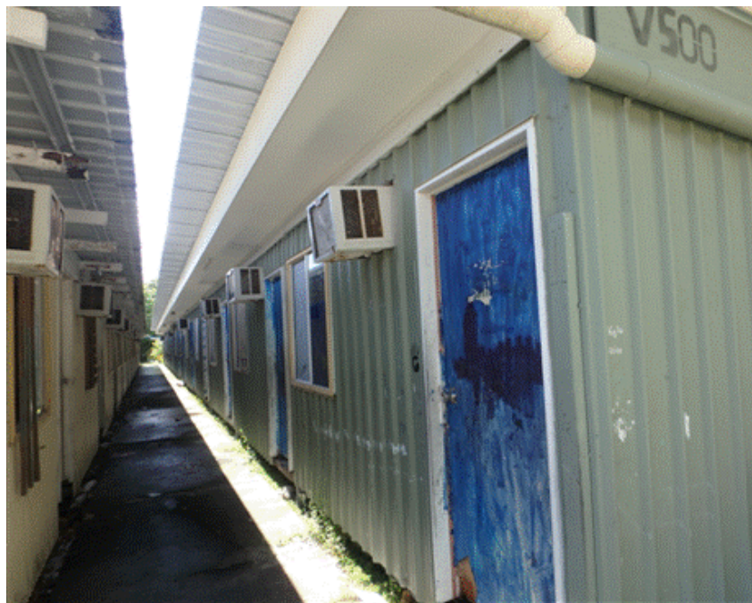
Figure B-5: Pre-fab buildings at Nauru Primary School in poor condition
