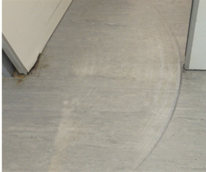
Figure B-11: Poor quality of construction at new hospital building where door frames are warping
