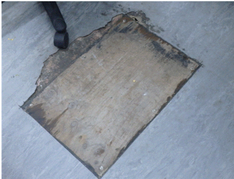
Figure B-10: Poor quality of construction at the new hospital building where floor tiles are lifting off
