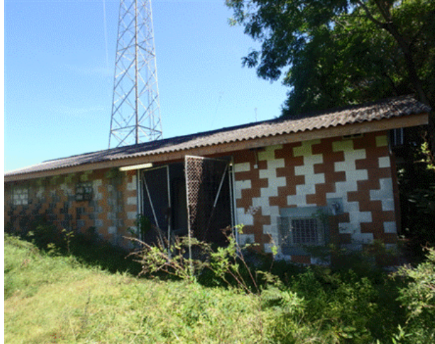
Figure B-15: Aviation equipment shed needs new roof and renovation
