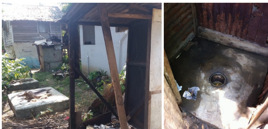
FIGURE 3.10: CLUSTER OF FUNCTIONING AND CLOSED PIT TOILETS IN BURNS CREEK NEAR HONIARA
