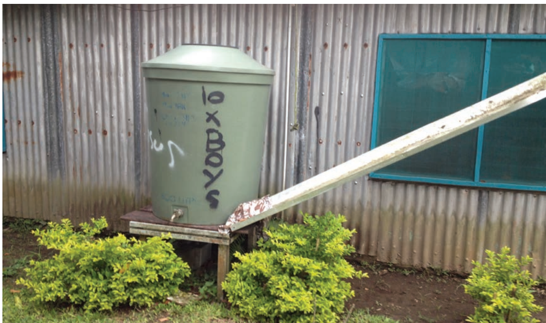
FIGURE 3.6: RAINWATER CATCHMENT CONTAINER IN BLACKSANDS SETTLEMENT IN VANUATU
