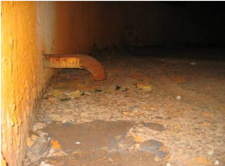
Corrosion of Decommissioned Water Storage Tank Floor.
