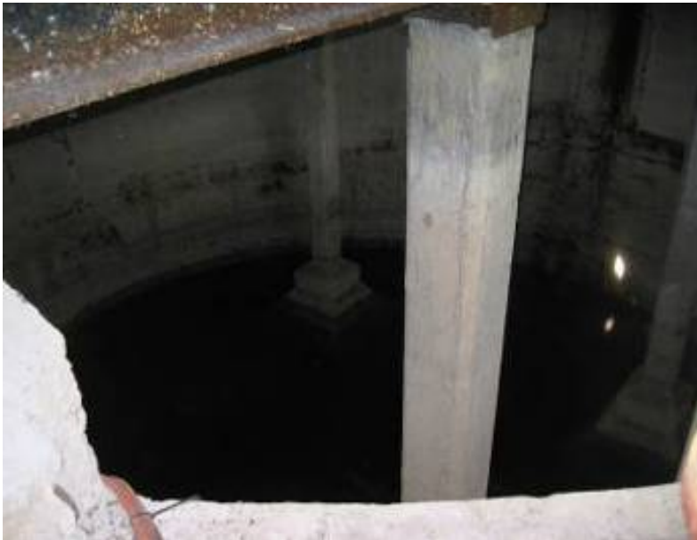
Rain Water Collection Tank.
