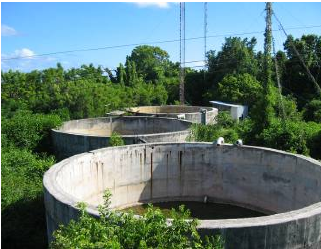
Sea Water Storage Tanks at Command Ridge.
