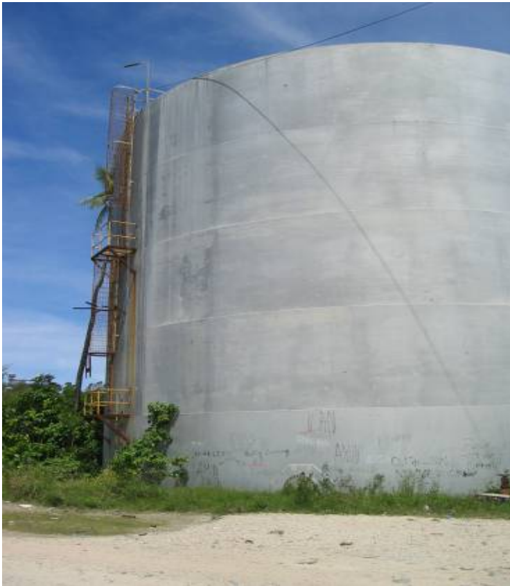
Potable Water Storage Tank B13.
