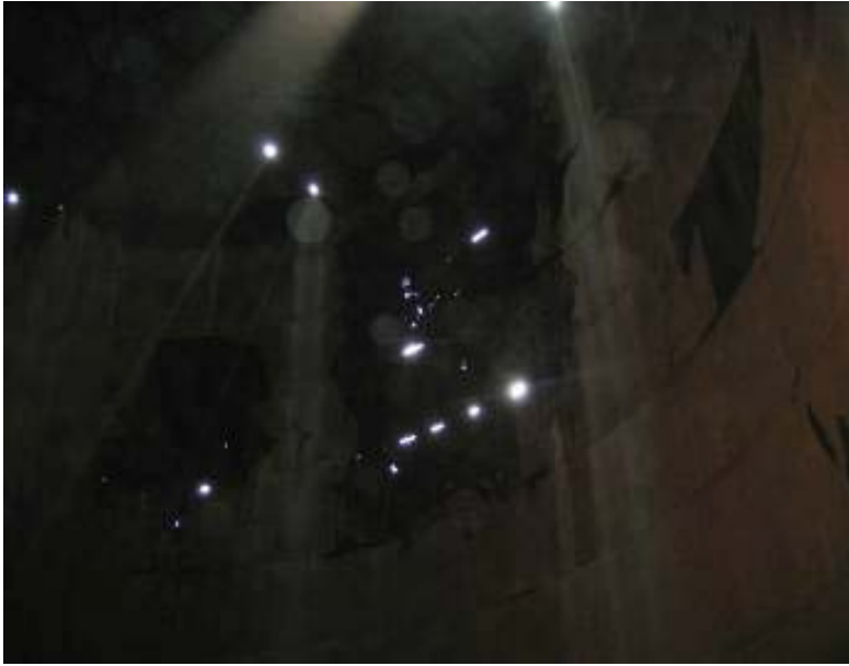
Corrosion in Decommissioned Water Storage Tank Walls.
