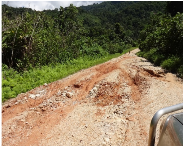
Figure 4. Typical erosion damage of long slope on East Road
