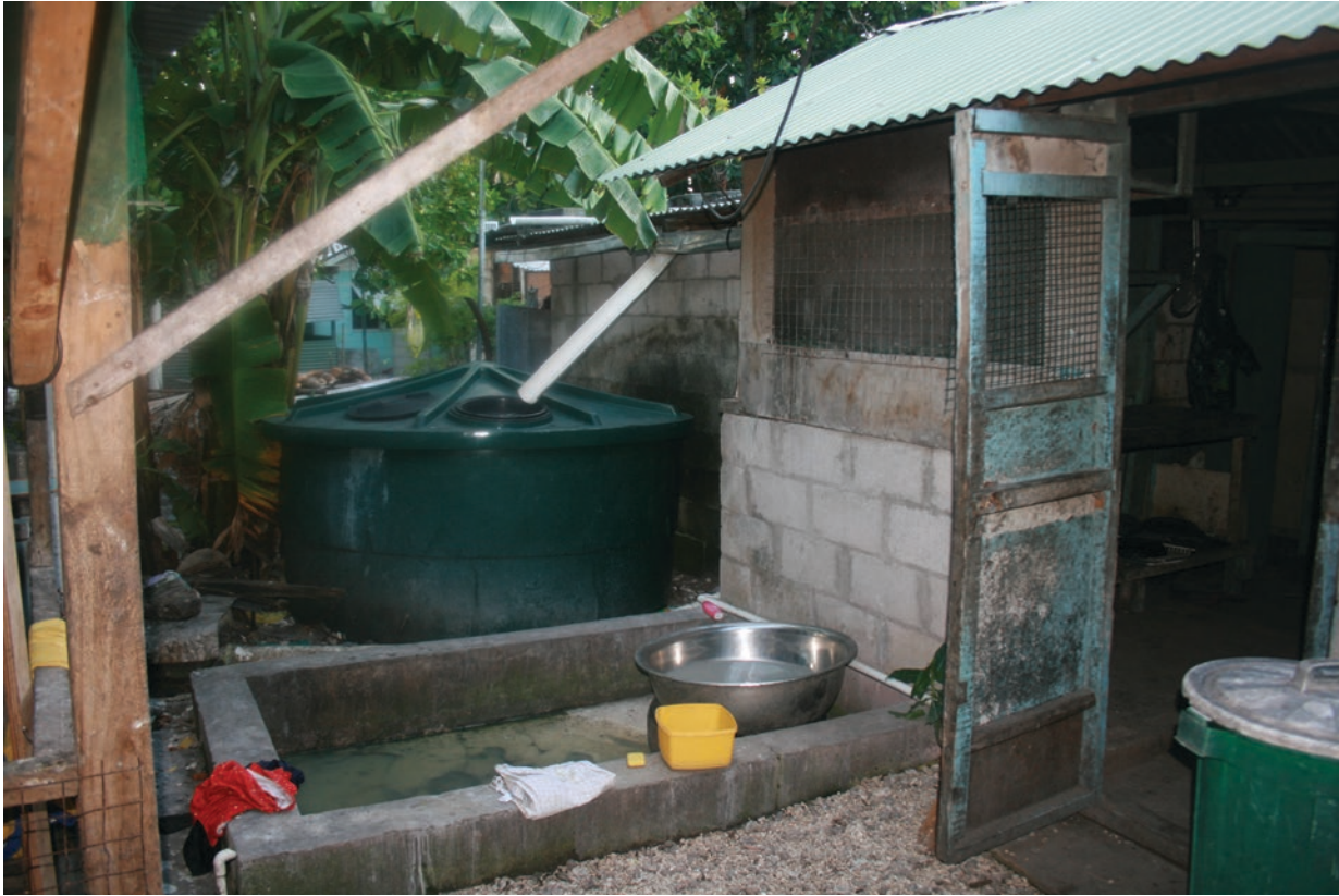
PHOTO 4.1. Private Rainwater Tank and Laundry Area
