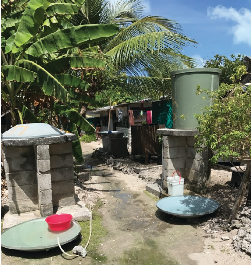
PHOTO 3.1. PUB Water Connection
