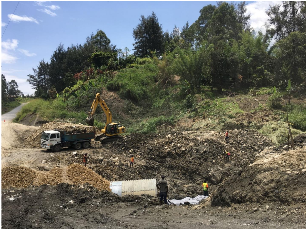
It is important to find ways to involve the private sector in providing and maintaining the country's infrastructure. Photo: David Ling.
