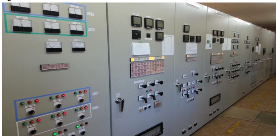
Figure 4.15: Switchboard at the PPUC
