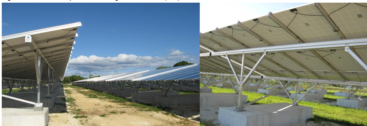
Figure A4.1 New Solar Operations at Tonga Power Limited (TPL)
