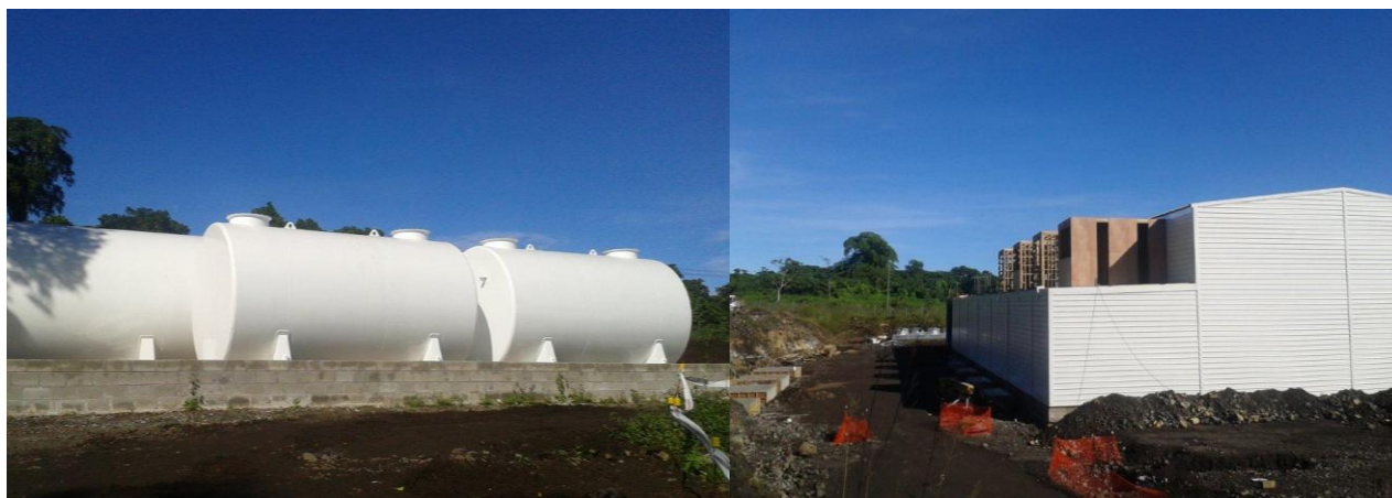
Figure 4.32: Diesel Tank and Power Plant at the Electric Power Corporation (EPC), Samoa
