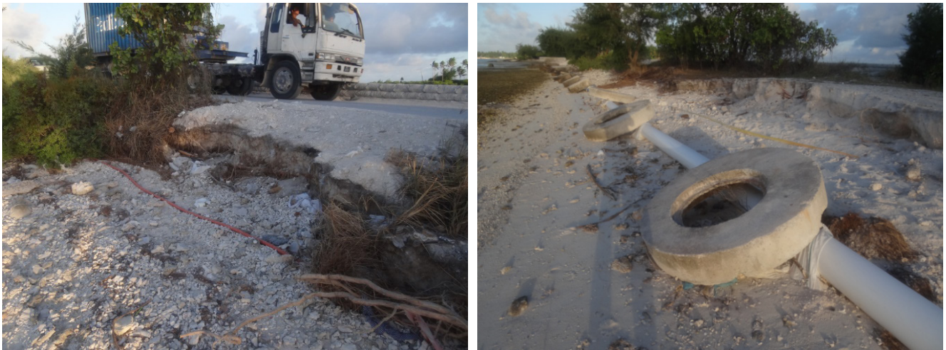
Erosion's dangerous effects. Coastal erosion is undermining roads (left) and utility infrastructure (right) in South Tarawa, Kiribati. Photo: Tom Shand.
