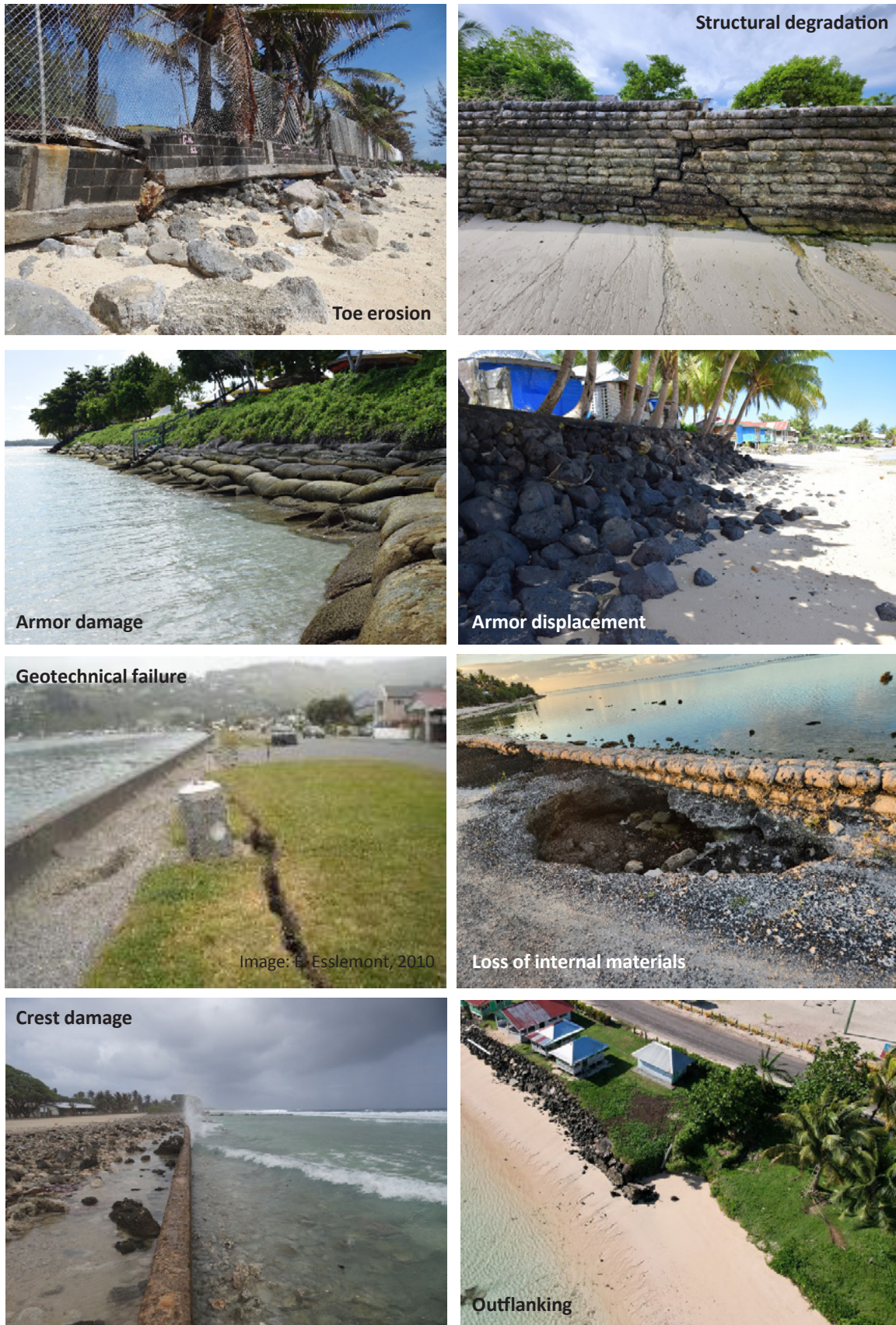
Figure 16: Examples of Typical Failure Mechanisms in Coastal Protection Works on Pacific Islands
