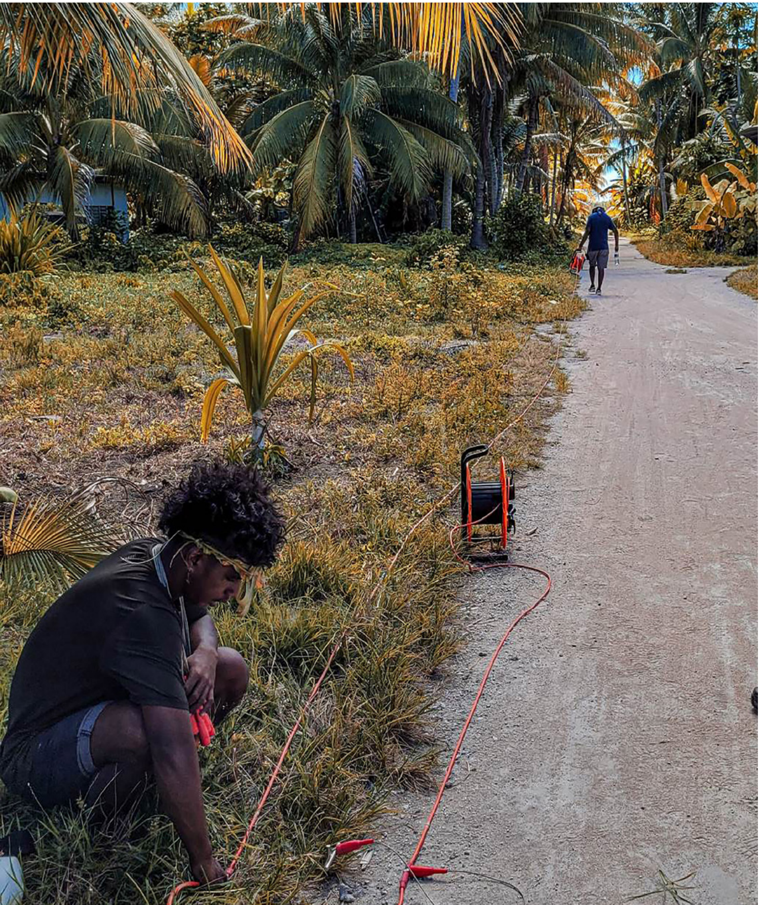
Workers on the renewable energy project in Nui, Tuvalu. Source: Tuvalu Red Cross.
