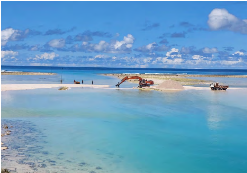
Figure 39: Clearing the Small Boat Channel in the Betio Bariki Causeway of Sand
