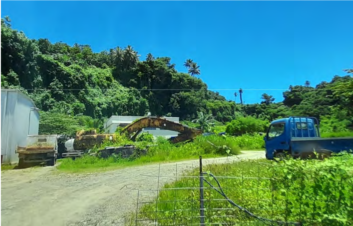
Figure 14. Rock Quarry Located Opposite the Kurrasa Hotel in Weno, Chuuk
