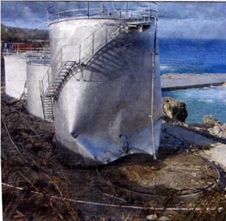
Figure: Existing Damaged Fuel Tanks and Tanktainers
