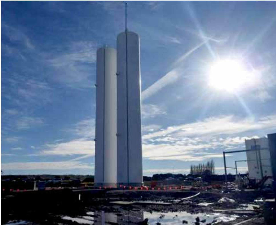
Figure 31. 300m 3 Cryogenic LNG Tank in Tasmania
