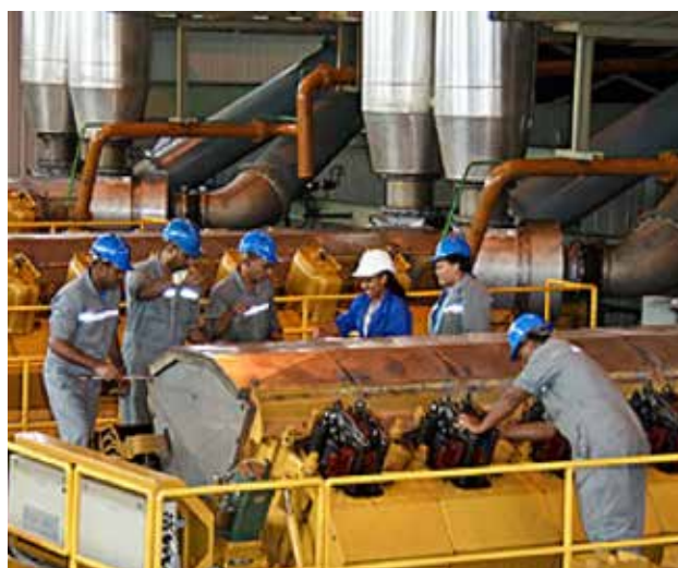
Figure C.1 Kinoya: Caterpillar Engines
