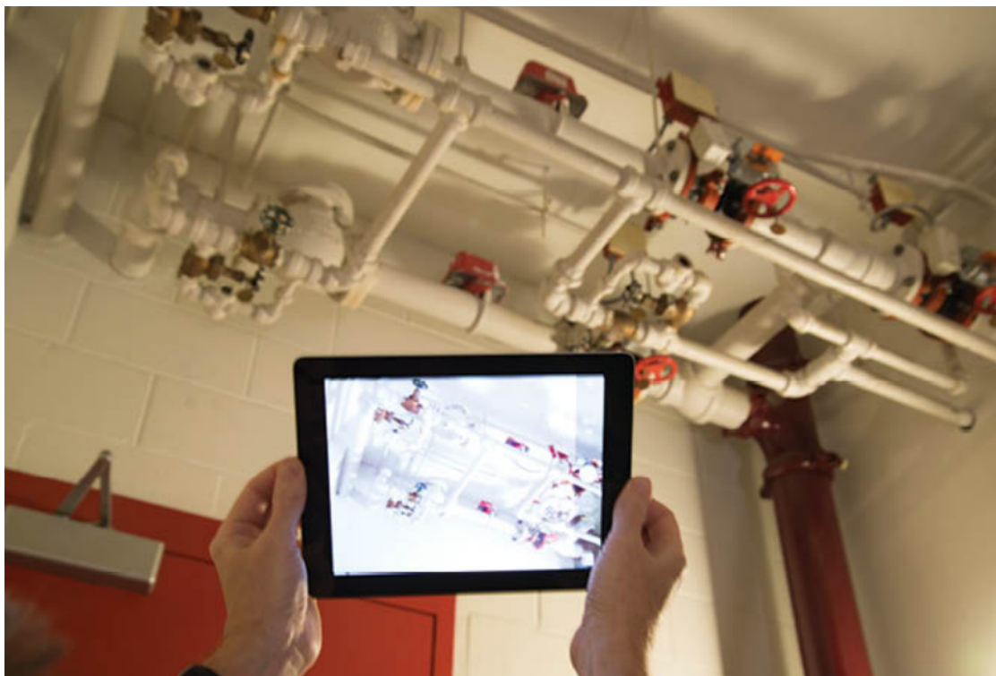
Figure 9: Fire System Piping Being Photographed on a Tablet in a Building Stairwell.
