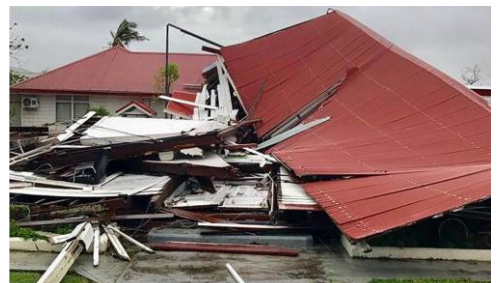
Tonga Parliament House. A local contractor is advising international experts on the reconstruction. (photo by BBC News).
