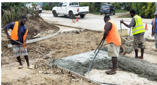
JCP slab under construction (note the poor Personal Protective Equipment). Espiritu Santo, Vanuatu. (Johnson 2018a).
