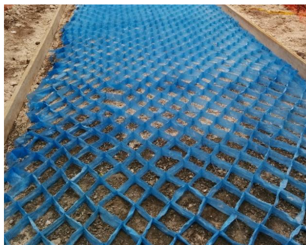
Geocell formwork expanded and tensioned and ready for placement of concrete (Whalley, O 2016).
