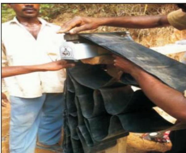
Strips of thick (>20 mm) geocell formwork (National Rural Roads Development Agency n.d., pg. 4).
