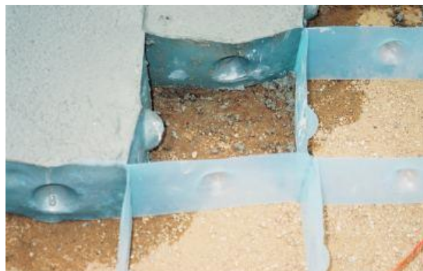
Dimpled formwork creates interlock between cells poured in situ (thin geocell formwork). (Hall & Hall 2007).
