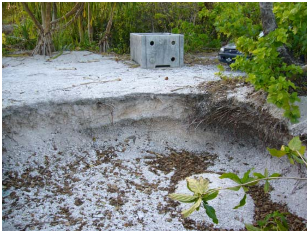
Figure 14. Sand and gravel mining has completely destroyed salinity monitoring borehole BN 16 (beside PS 7), one of the oldest and the deepest borehole in Bonriki.
