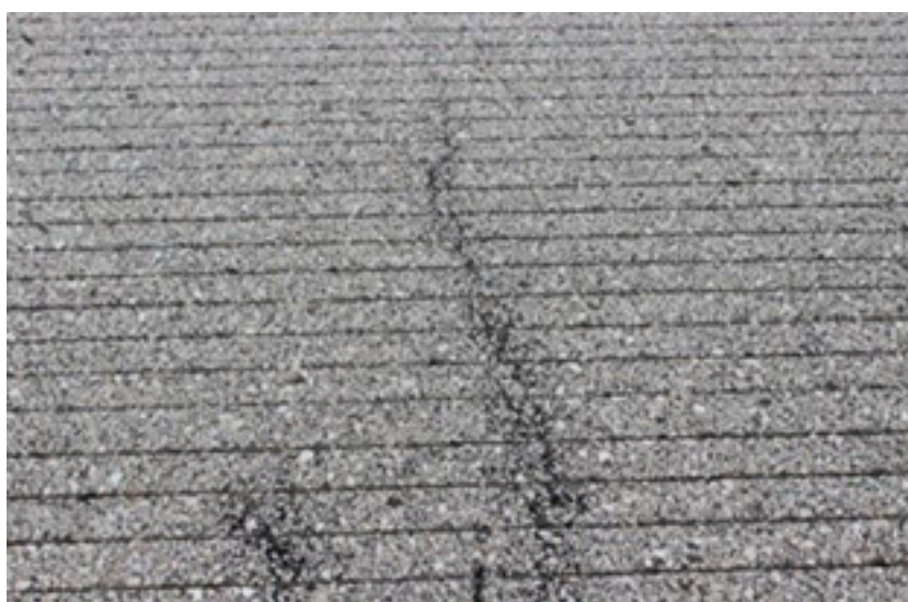
Figure 8-1: Runway Surface Degradation due to Cracks
