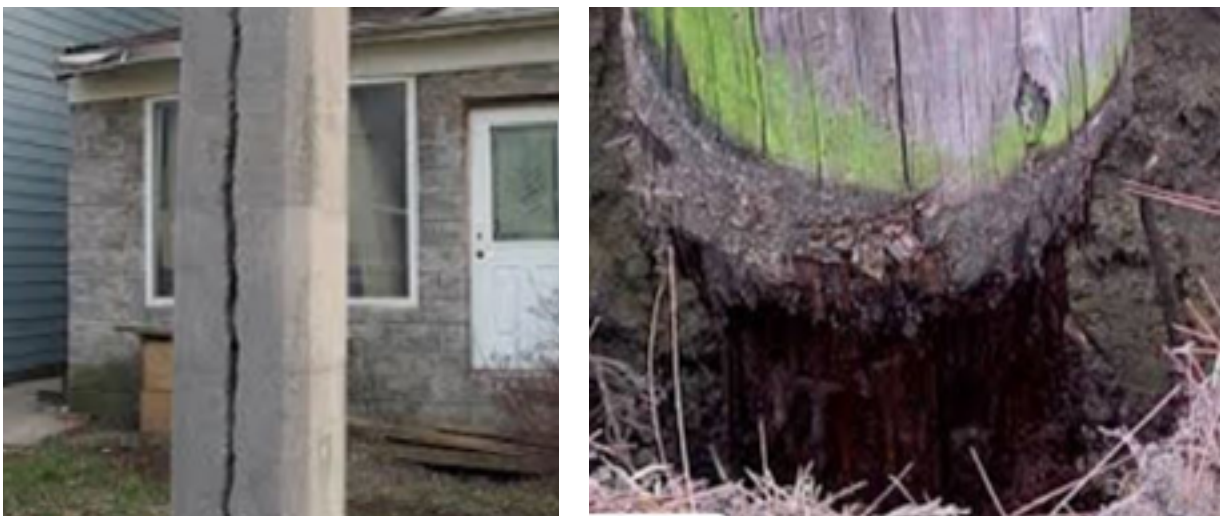
Figure 12-7: Overhead Line Poles in Poor Condition
