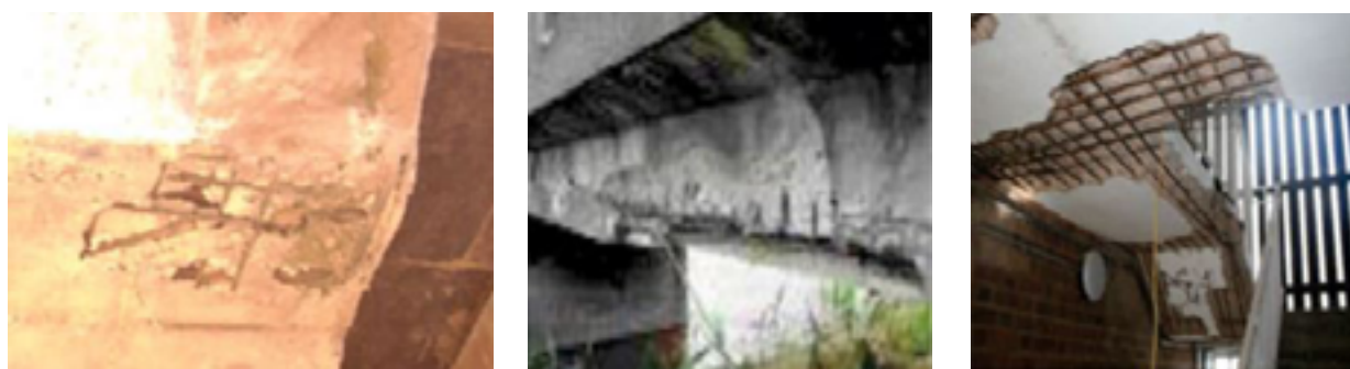
Figure 7-5: Degradation of Concrete in Bridges
