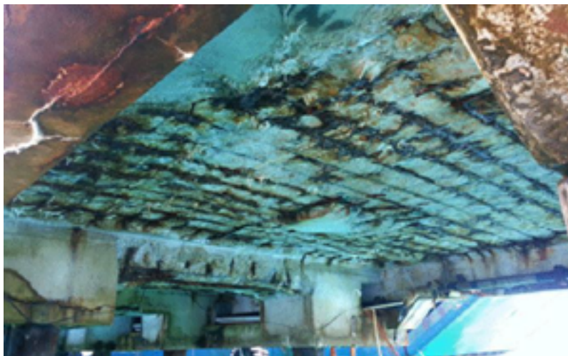
Figure 9-2: Concrete Structure in Very Poor (Badly Corroded and Rebar Exposed)
