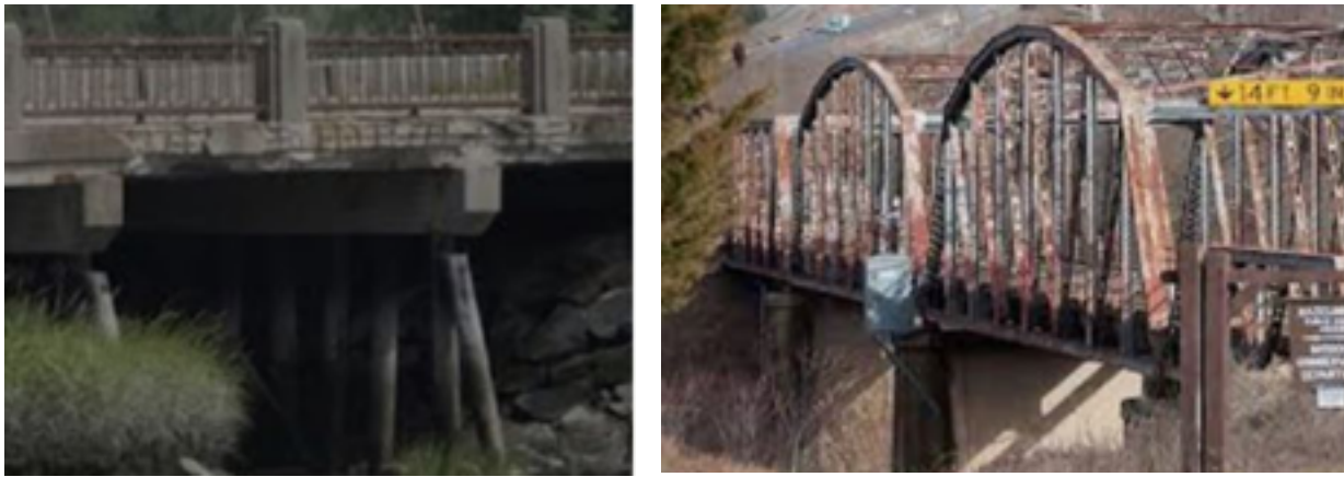
Figure 7-6: Bridges in Poor Condition
