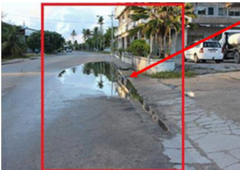
Figure 6-4: Degradation Modes—Clogged Drainage Sump
