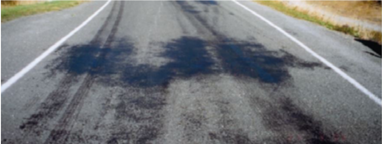
Figure 6-3: Degradation Modes of Chip Seal Roads—Bleeding and Tracking
