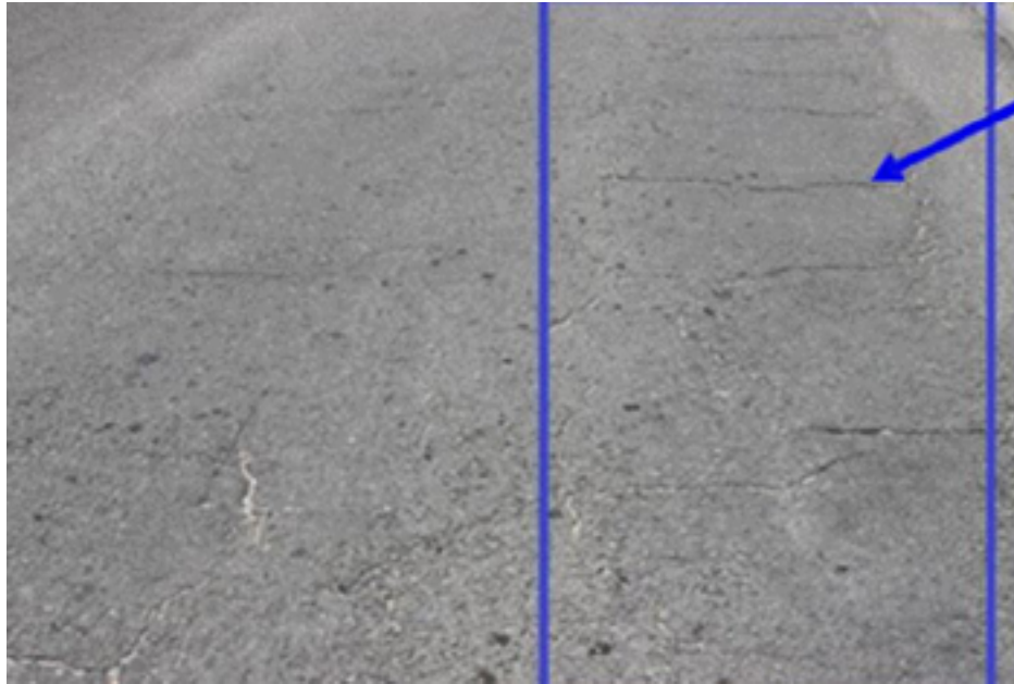
Figure 6-1: Road Degradation Modes—Surface Cracks
