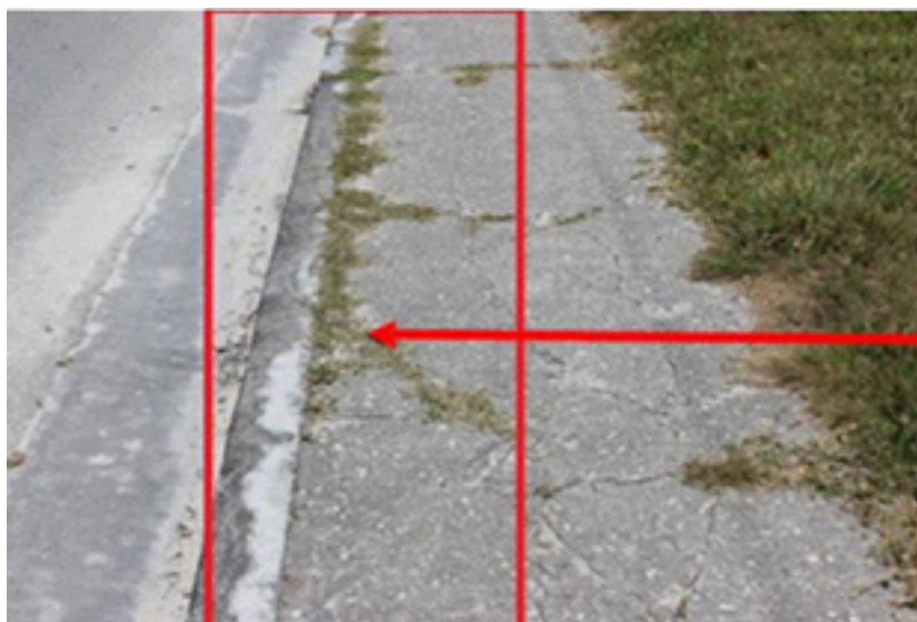
Figure 6-5: Degradation Modes of Concrete Footpath
