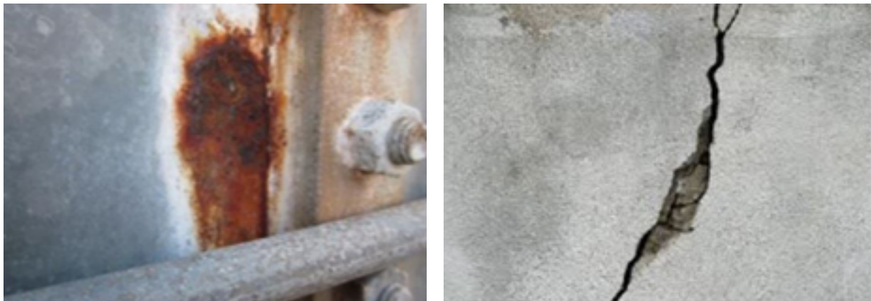
Figure 11-12: Water Storage Tanks in Poor Condition
