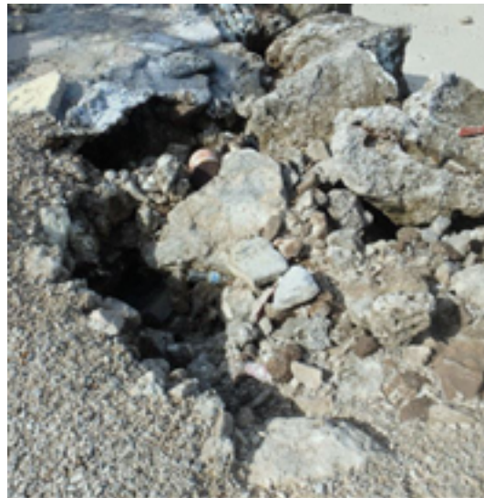
Figure 10-4: Rock Revetment in “Poor” Condition due to Erosion
