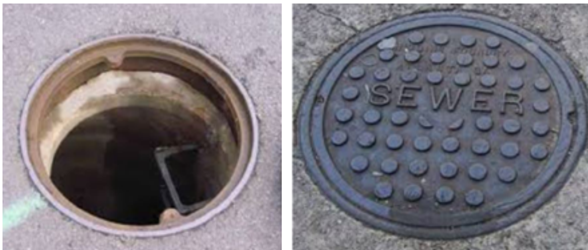
Figure 11-7: Sanitary Sewer Manhole
