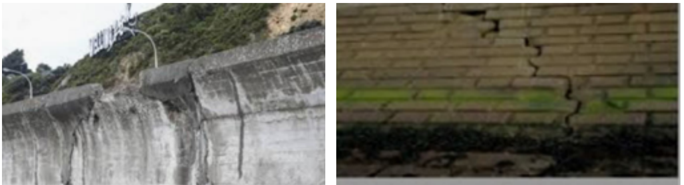
Figure 10-3: Seawalls in “Poor” Condition due to Structural Damage
