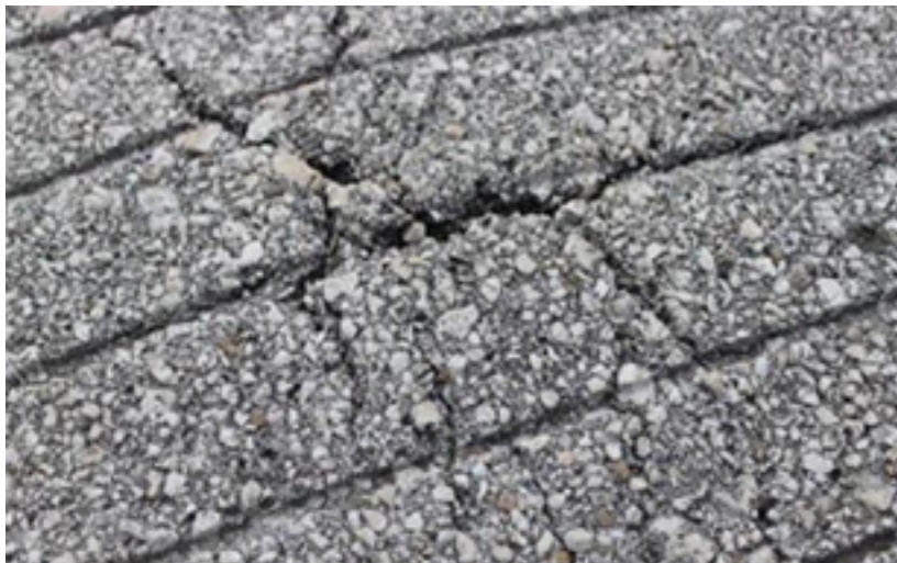
Figure 8-3: Runway Surface Degradation due to Volcano Cracks
