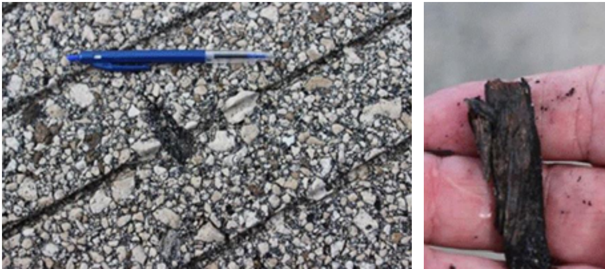
Figure 8-2: Runway Surface Degradation due to Vegetation Plucking-Out
