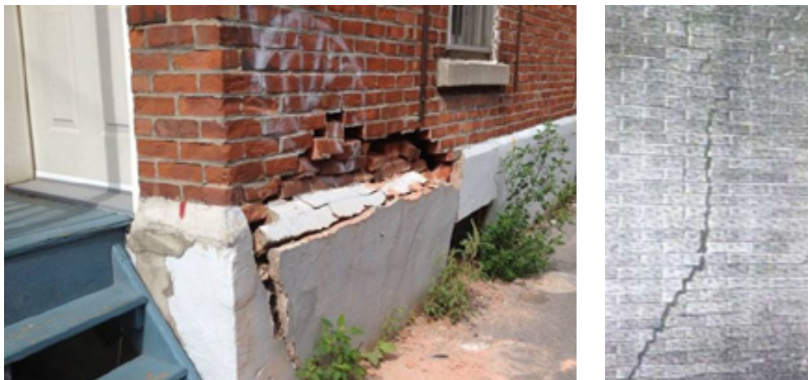
Figure 5-3: Structural Cracks in Masonry
