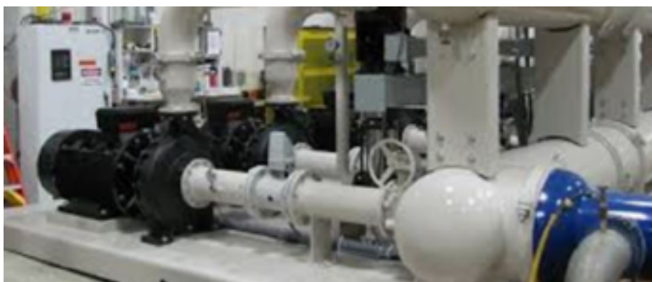
Figure 11-5: Water Pumping Station
