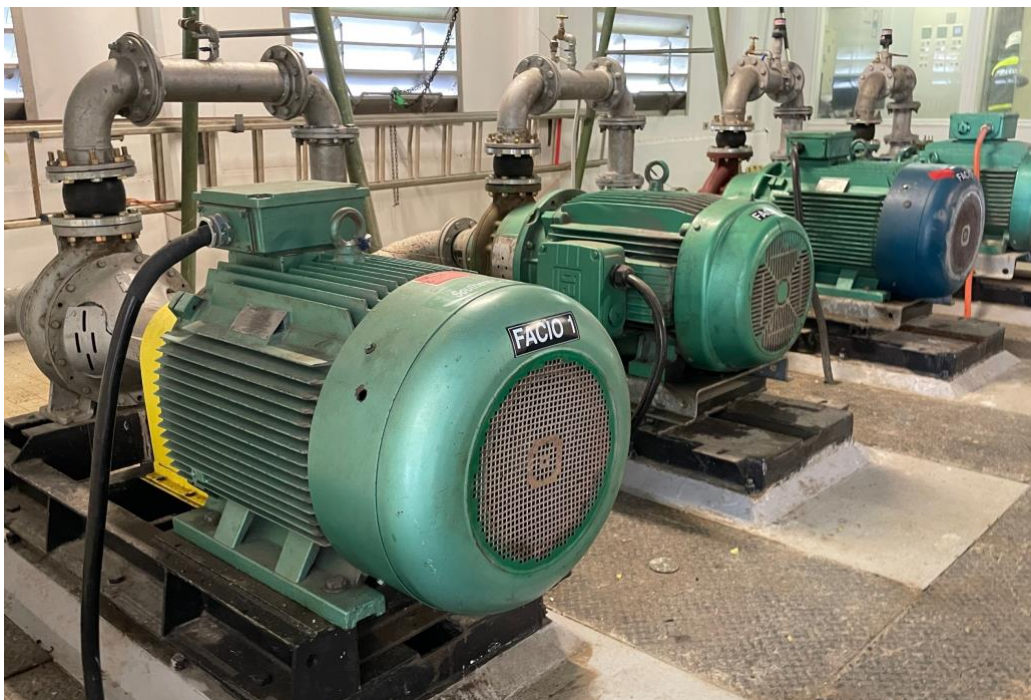
Water distribution pumps, Vanuatu
