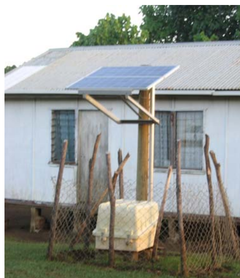
Figure 9. Household PV System located on 'O'ua Island, Tonga.
