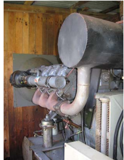
Figure 22. Biofuel generator, Vanua Balavu, Fiji.
