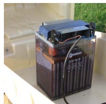
Figure 10. PV System battery.
