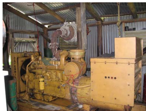
Figure 5. Diesel generator, Vanua Balavu, Fiji.
