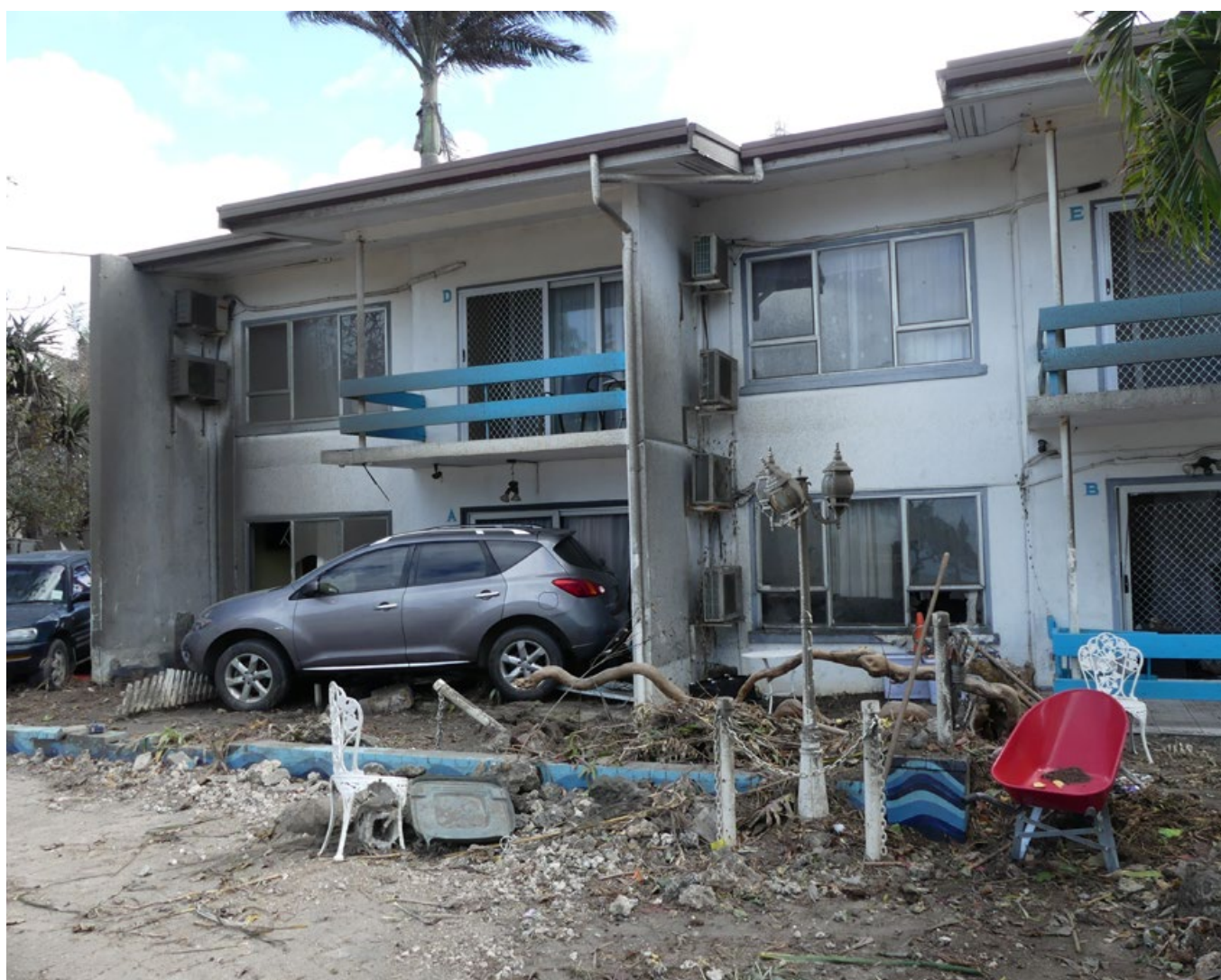
Sopu Captain Cooks Apartment - car on verandah
