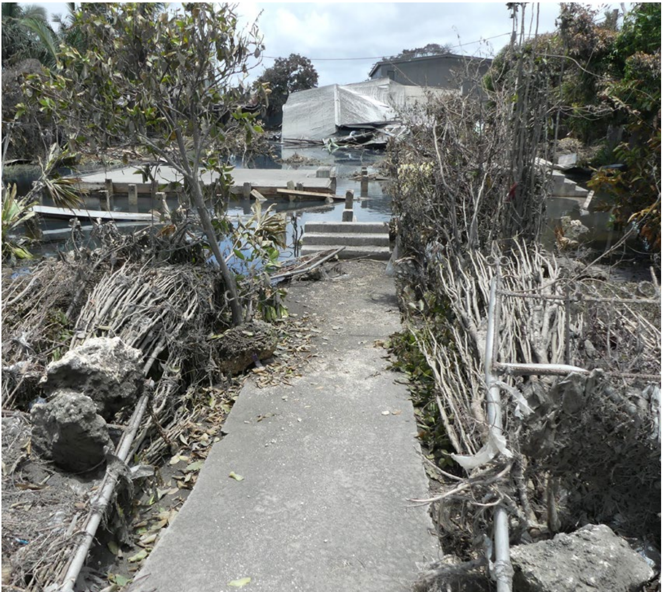
Vuna Road house washed from base, crushed at back.
